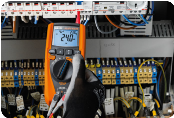
RCD tripping time and current measurement.
