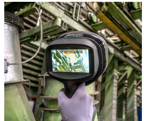
The FLIR Si2-LD detects two sources of potential compressed air leaks, distinguished from background noise.
